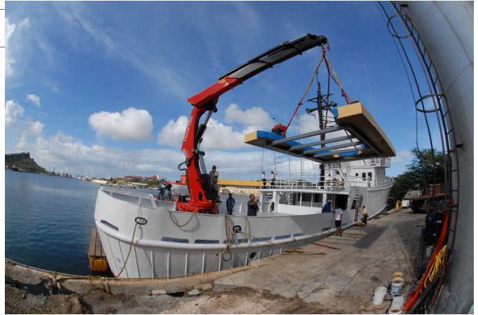
The big Fassi crane easily lifts the docking platform from the ship into the water.
